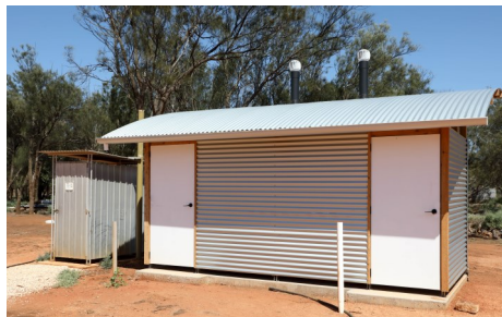
New toilet block by Visitors Centre nears completion. These facilities also cater for disabled visitors. Note the old adjacent toilet that has served Gluepot for nearly 25 years. This is soon to be removed.
